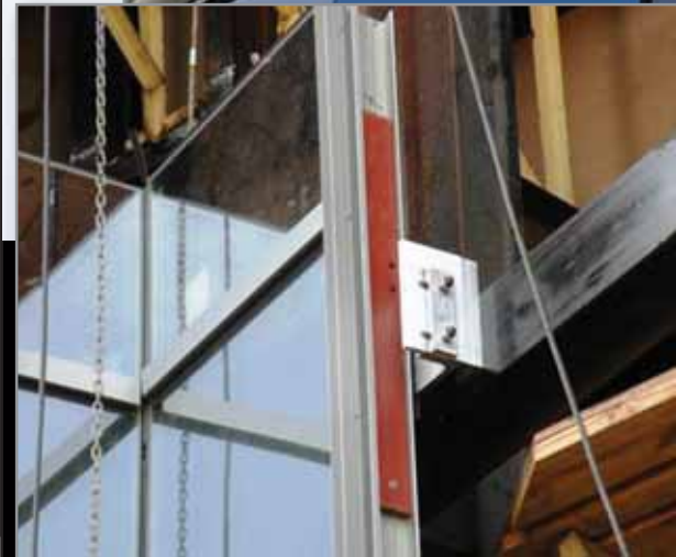
An anchor designed for a custom unitized curtainwall system is used to attach the curtainwall back to structure.
